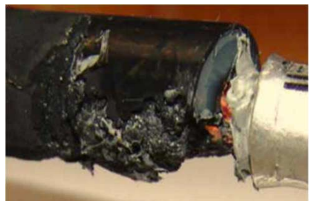
Fig.8: Immediate failure due to insulation screen not being removed during installation [16].
