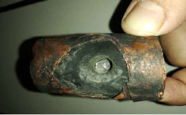
Fig.1: The cable insulation breakdown by the treeing process due to existence of air voids or impurities inside the insulating material.
