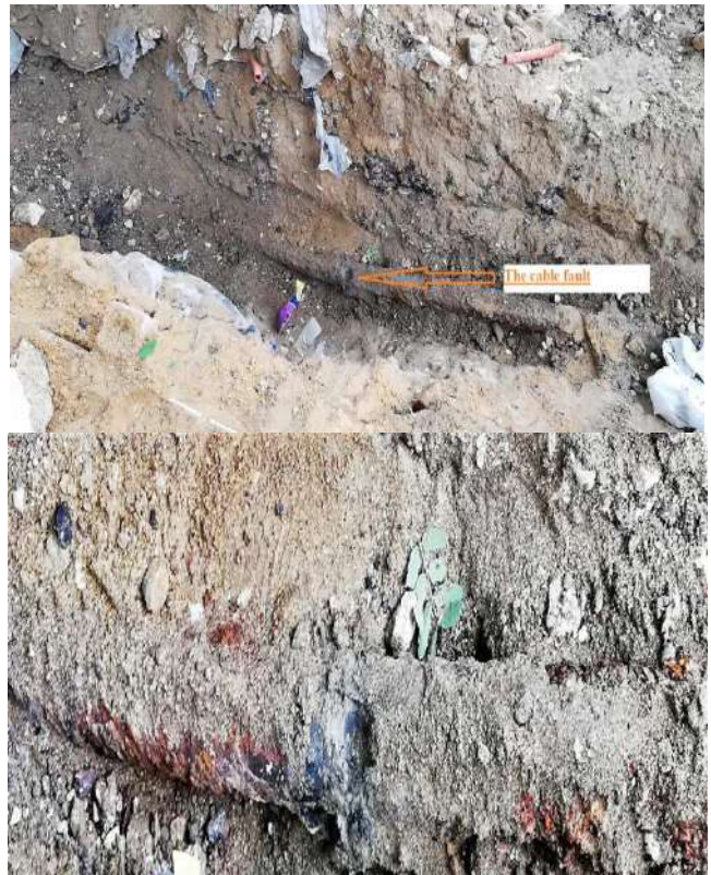
Fig.2: Oil impregnated paper cable insulation breakdown due to aging and existence of old digging process beside it.
