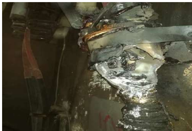
Fig.10: The expulsion of oil impregnated paper oil filled termination.
