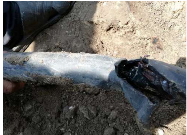
Fig.11: The cable mechanical fault by mechanical digging instrument.
