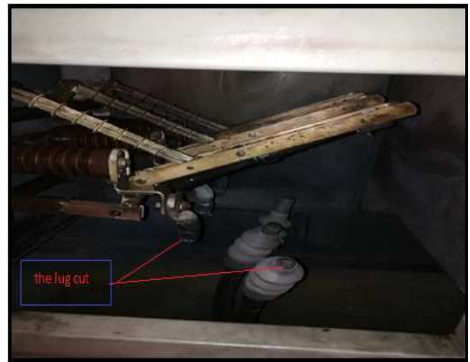
Fig12: The destruction of the termination lugs.
