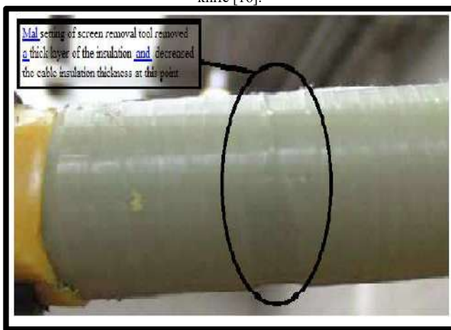
Fig.5: Extremely rough insulation surface resulting from incorrect setting and/or misuse of screen removal tool [16].
